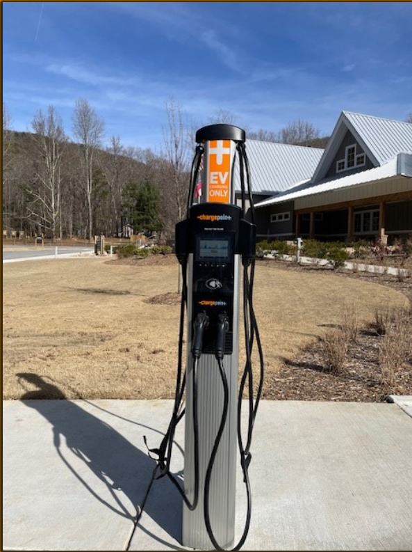
An EV charging station is now available.
