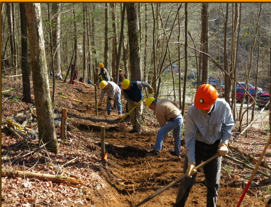
Tom leading the way on construction of the Fall Branch Falls Reroute.
