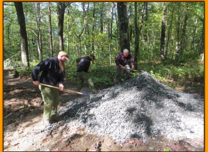
Two Forest Service personnel and BMTA's David Ricker start shoveling and then spreading gravel.
