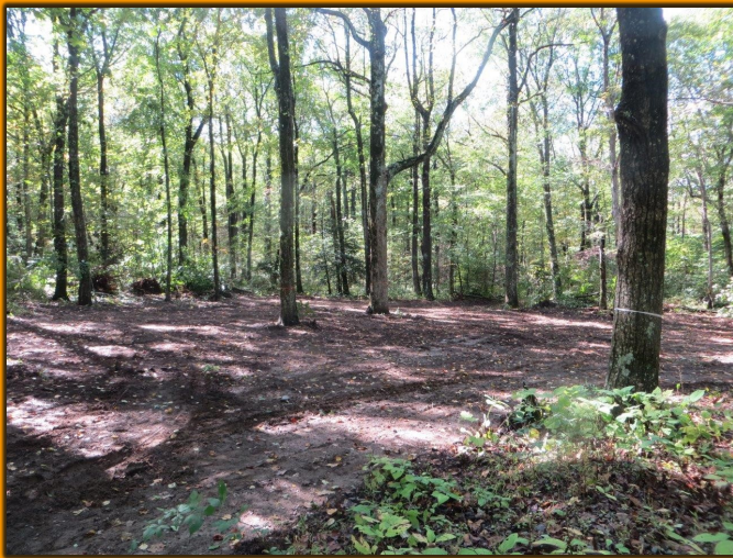
Our new BMT Springer Mountain parking lot stands cleared awaiting the first gravel truck.
