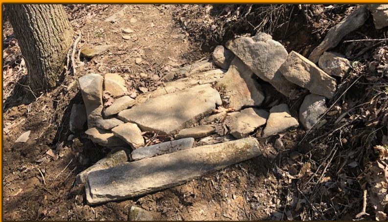
A seep crossing architected and built by Steve Bayliss...allows the water to run under the rocks versus across the trail. (credit: Debra Guhl)
