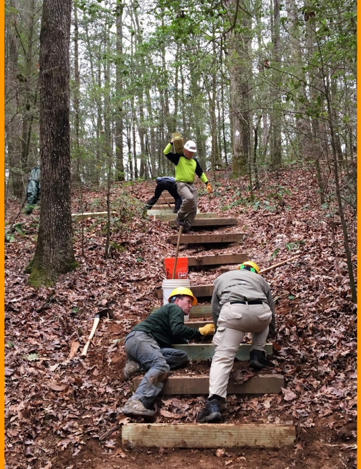
Installing new steps: Top L to R – Russ Johnson, Brian Trinkle Bottom, L to R – Bob Cowdrick and Mike Kovitch.
