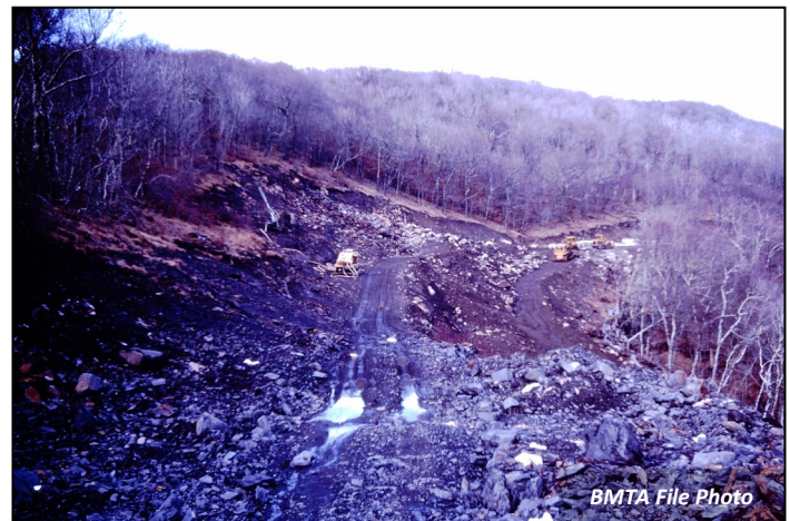
January 8, 1989. There was a brief scouting trip that started on the east side of Haw Knob, just into North Carolina and about a mile from Mud Gap where the Benton MacKaye Trail is now located. This picture shows the construction of the Cherokee Skyway. There was an existing trail, the Hooper Bald Trail, that ran from Mud Gap over Haw Knob and Big Junction to Hooper Bald, well east of the current Benton MacKaye Trail route. The Skyway was superimposed on parts of this old trail.
